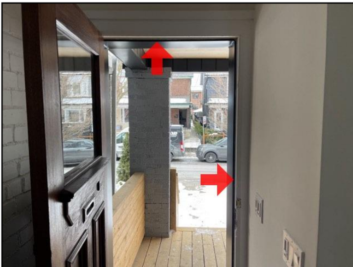
28. Weatherstripping missing or ineffective
