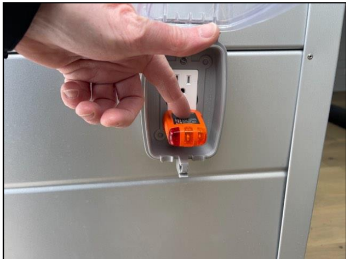
5. GFCI/GFI needed (Ground Fault Circuit...
