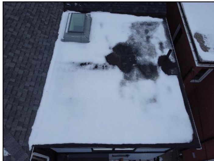
1. Due to excess snow and ice coverage on roof...
